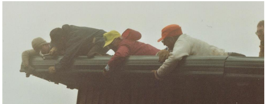
Replacing the roof on Cooper Lodge inside a cloud in the early 1980s.
